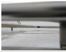
Aerial, Broken, Replace
