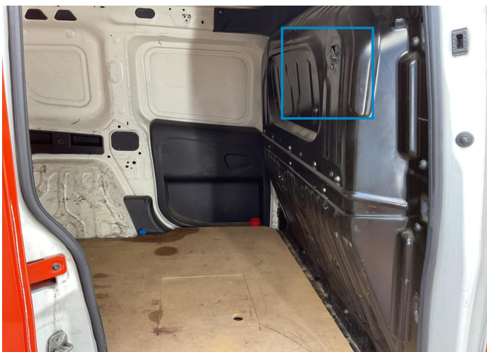
25. Cabin Interior / Broken -
