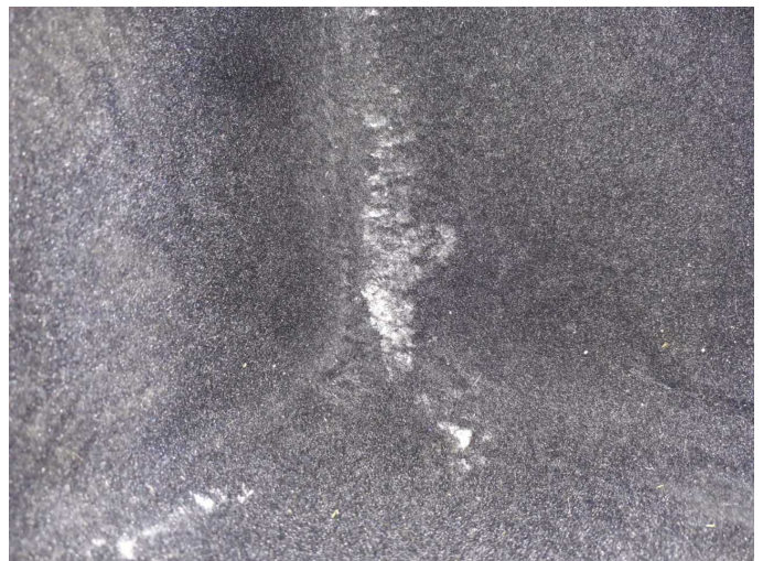
Damage 8: Interior: Interior (Schimmelbildung) - Soiled - Clean
