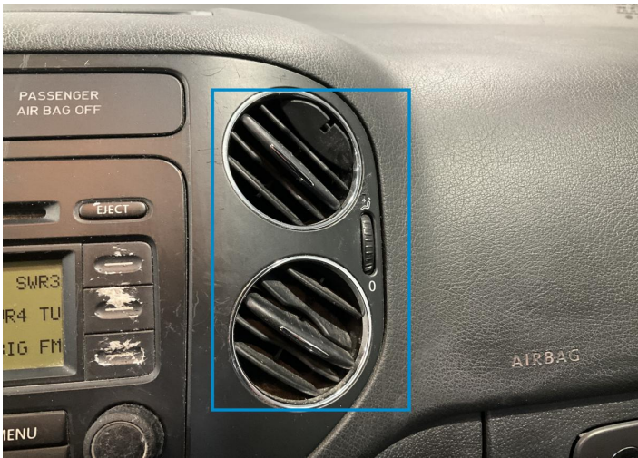
5. Aeration Grid / Front Center Interior / Not Working -
