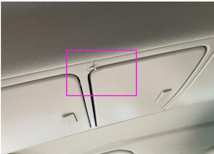
33. Roof Upholstery Interior / Broken -
