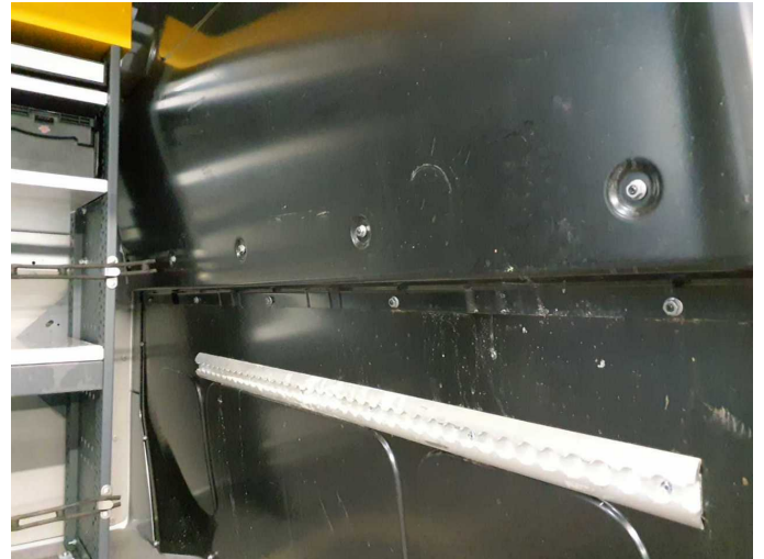
Wear and tear 2: Body: Partition wall (Dellen) - Scratched - No deduction
