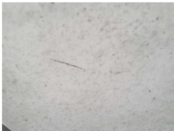
Wear and tear 6: Roof: Roof (Kofferaufbau, von innen sichtbar) - Scratch(es) - No deduction
