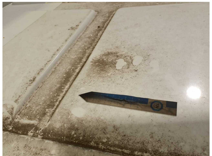
Damage 7: Roof: Roof - Corrosion - Repair and paint
