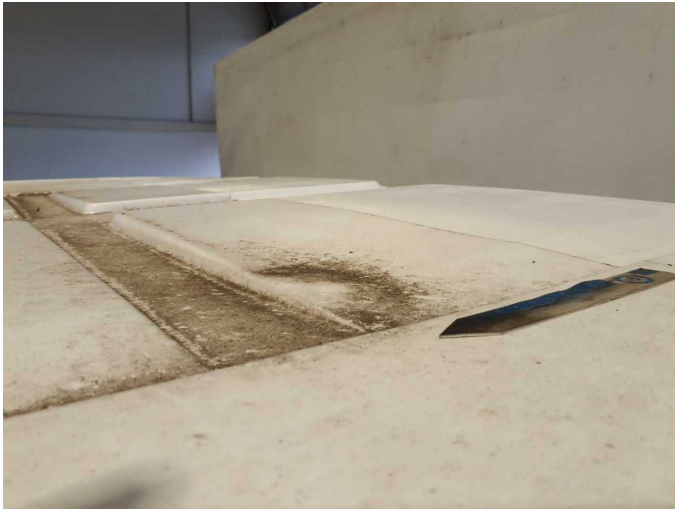
Damage 7: Roof: Roof - Corrosion - Repair and paint
