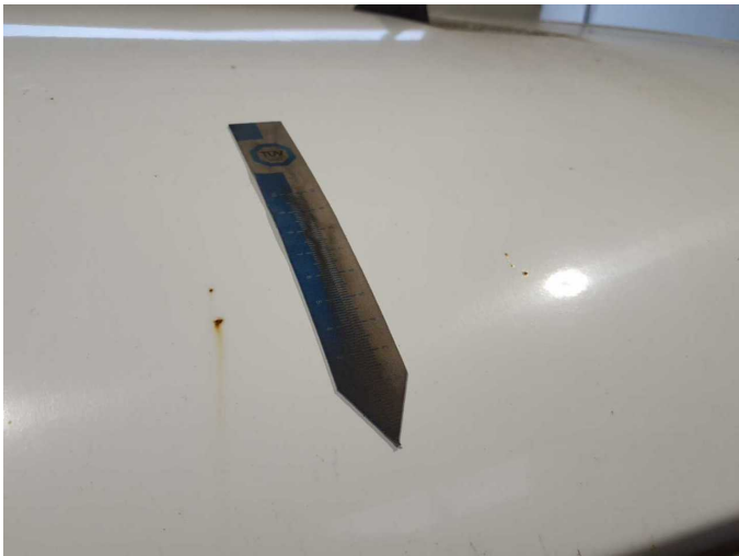
Damage 7: Roof: Roof - Corrosion - Repair and paint
