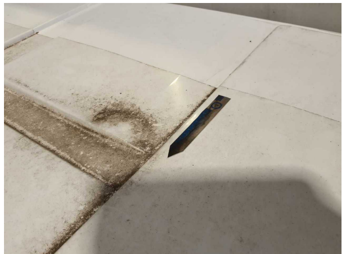
Damage 7: Roof: Roof - Corrosion - Repair and paint
