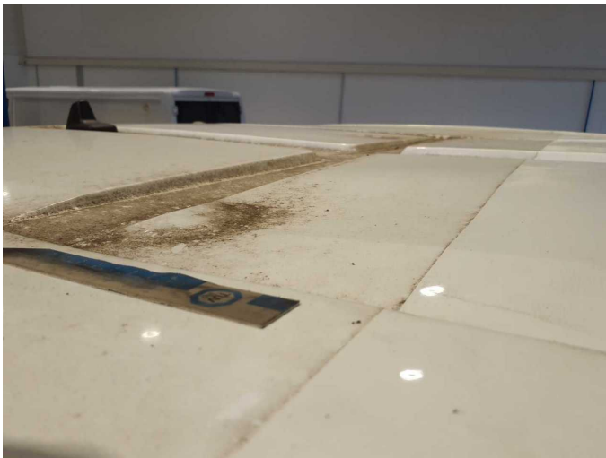
Damage 7: Roof: Roof - Corrosion - Repair and paint
