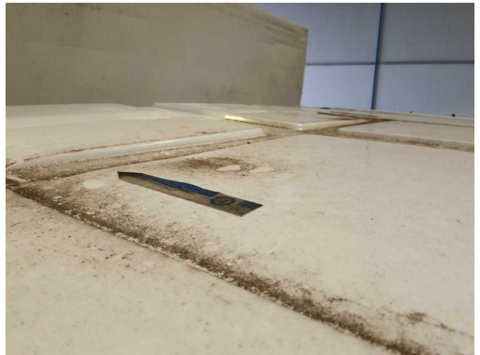
Damage 7: Roof: Roof - Corrosion - Repair and paint
