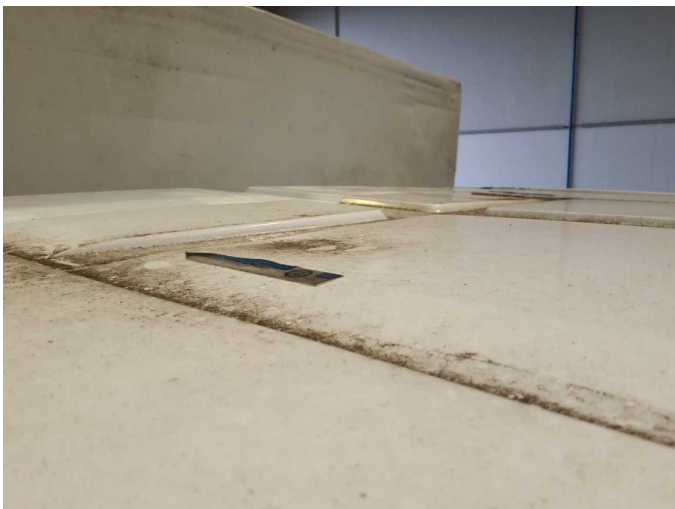
Damage 7: Roof: Roof - Corrosion - Repair and paint
