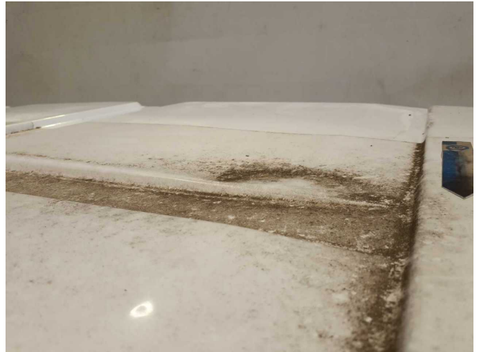
Damage 7: Roof: Roof - Corrosion - Repair and paint
