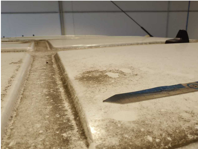
Damage 7: Roof: Roof - Corrosion - Repair and paint
