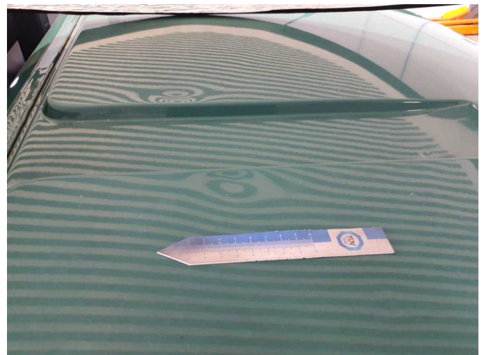
Damage 15: Roof: Roof - Deformed - Repair and paint
