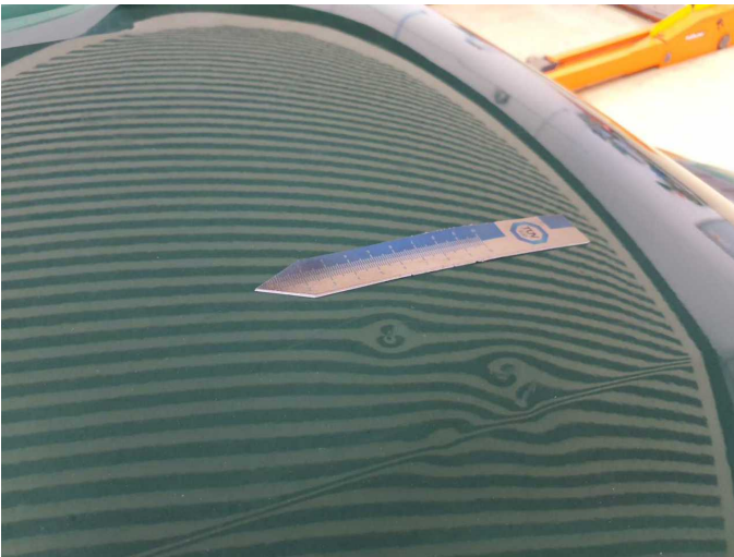
Damage 15: Roof: Roof - Deformed - Repair and paint
