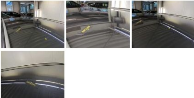
Roof, Hail damage, Paintless dent repair (hail)
