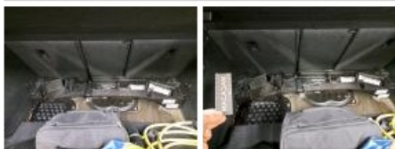
Charging cable (normal), Missing, Replace
