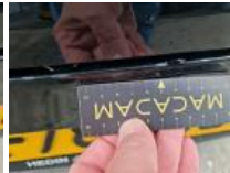
Roof, Chemical polution, Polish
