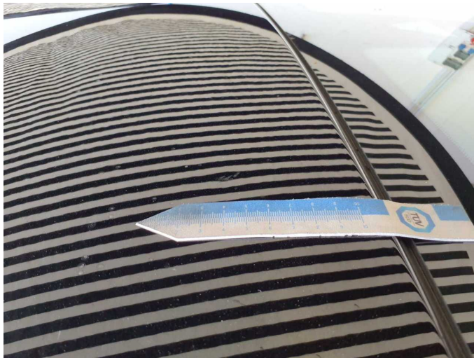
Damage 3: Roof: Roof - dent(s) - Smooth repair work
