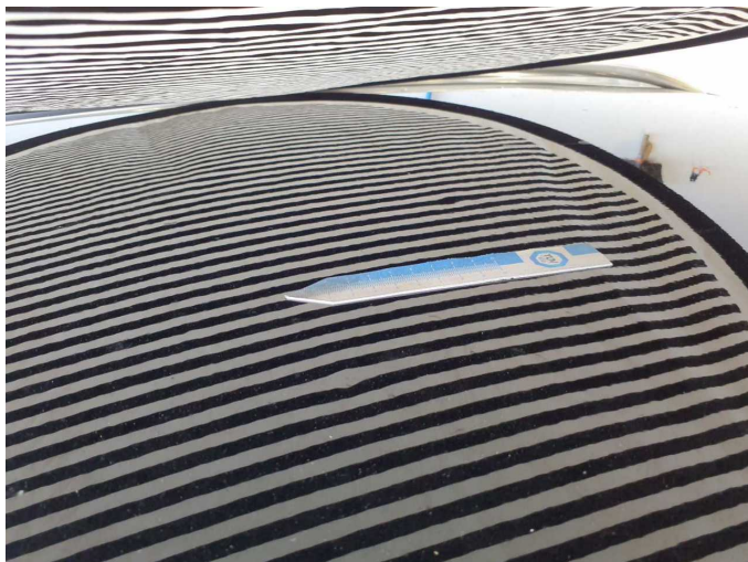
Damage 3: Roof: Roof - dent(s) - Smooth repair work
