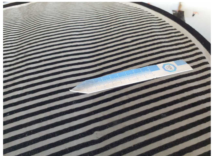
Damage 3: Roof: Roof - dent(s) - Smooth repair work
