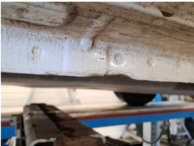
Damage 14: Sill - right side: Sill - Deformed - Repair and paint
