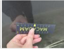
Roof, Chemical polution, Polish
