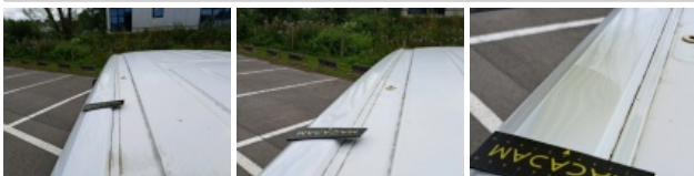
Steel rim FL, Rust, Acceptable
