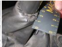
Floor covering R, Damaged, Replace
