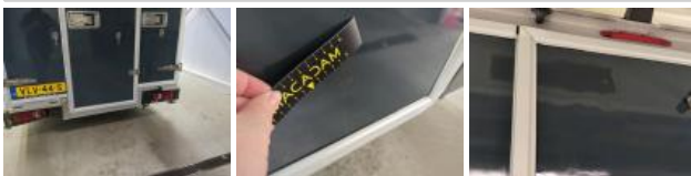
Boot door panel RR, Crack, Repair and paint (complete)
