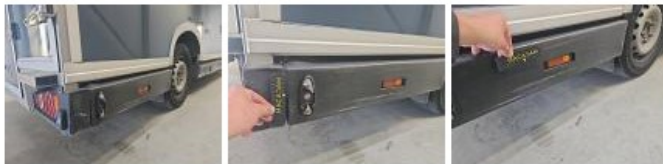
Shutter / cover R, Deformed / Strained, Replace
