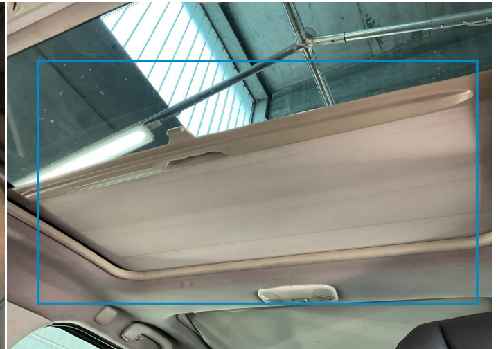
4. Roof Upholstery Interior / Broken -
