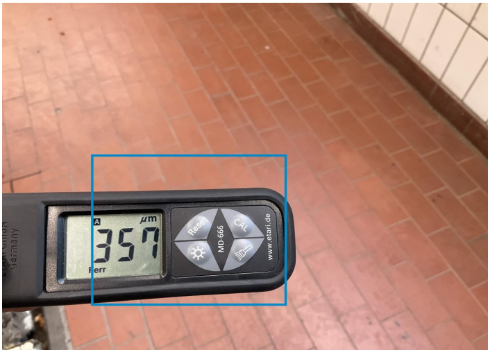
5. Door / Back Right Paint / Poor Previous Repair -
