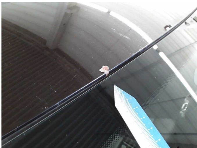
Damage 10: Roof: Roof - Corrosion - Paint
