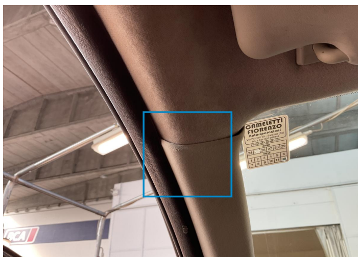
37. Roof Upholstery Interior / Ripped -
