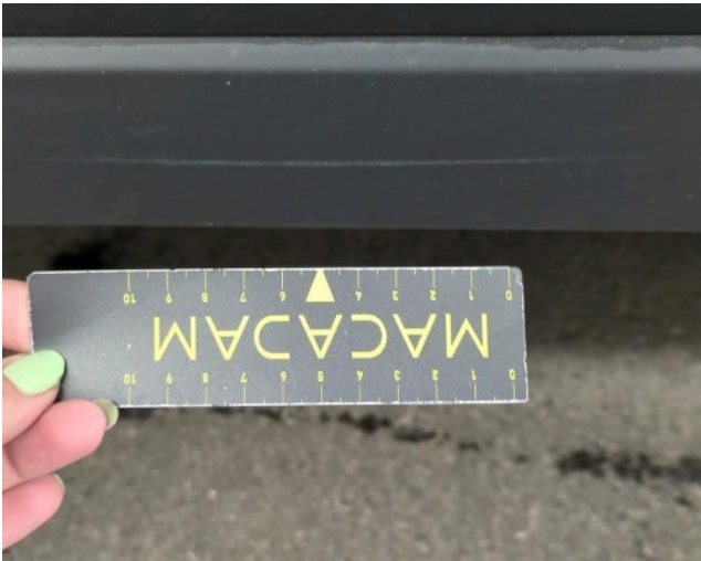
No extra information about this damage.
