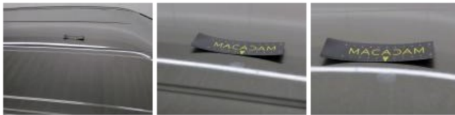
Roof, Chemical polution, Polish
